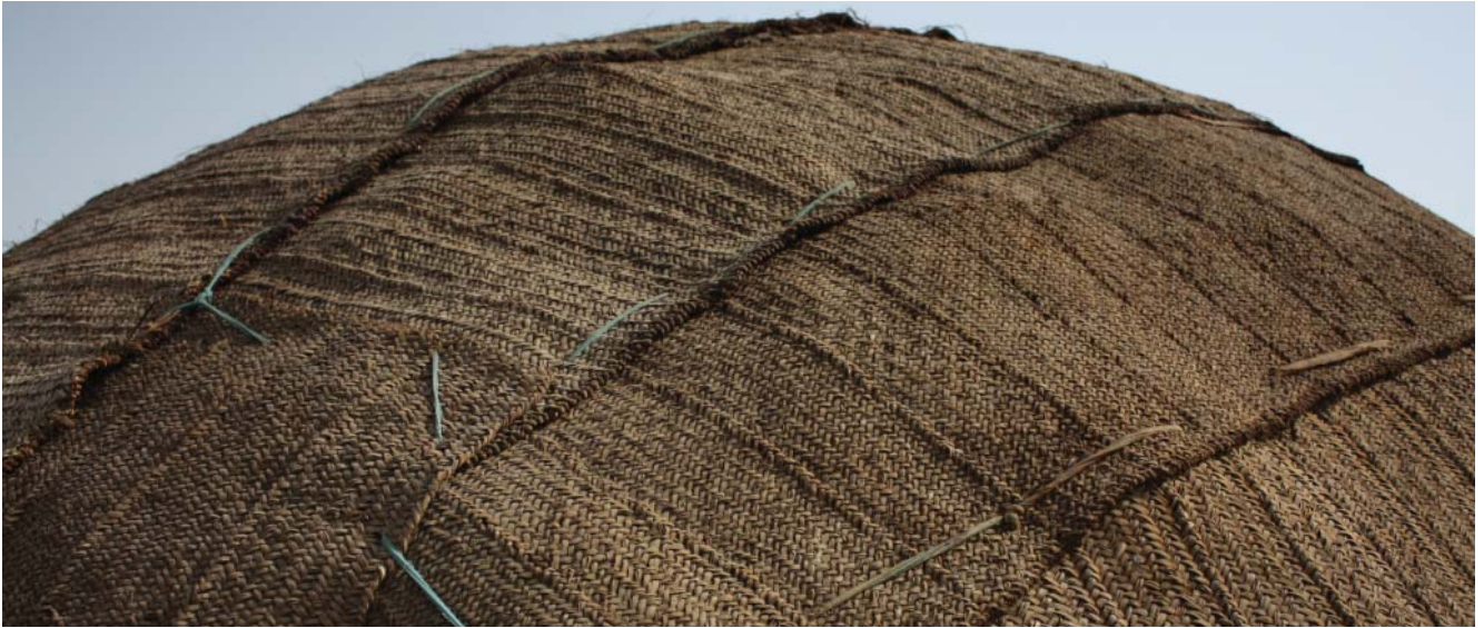
Fig. 263: mats of the cover are arranged from the bottom to the top of the framework with sufficient overlap foreseen for each layer of mats
