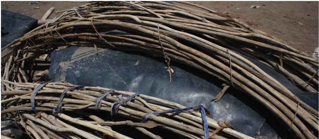
Fig. 248: halawwa - members of the armature are gathered or cut when they are green and still easy to bend while constructing a house; with time they dry slowly till a natural yield is created and members remain in form of arches
