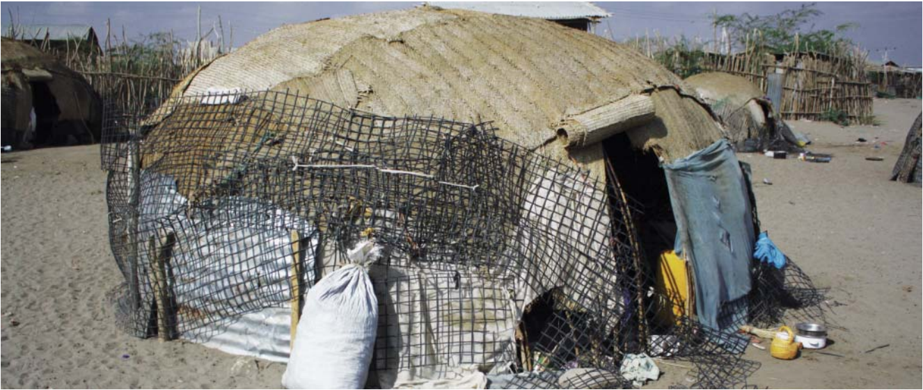
Fig. 227: Logya, Dubti woreda: hemispherical daboyta with a roof slightly collapsing under own weight due to too slender diameter of members
