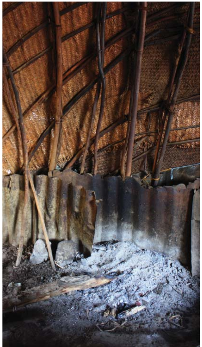
Fig. 359: the construction of the tent is covered with metal sheets, which protect it from catching fire
