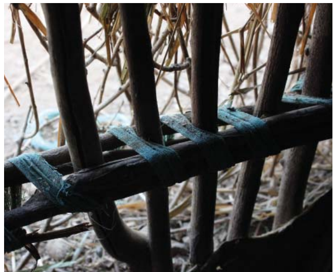
Fig. 308: Gubiyra, Yalo woreda : lower parts of grass hut are left open for ventilation; at night the lower part is covered with mats, foils or stones
