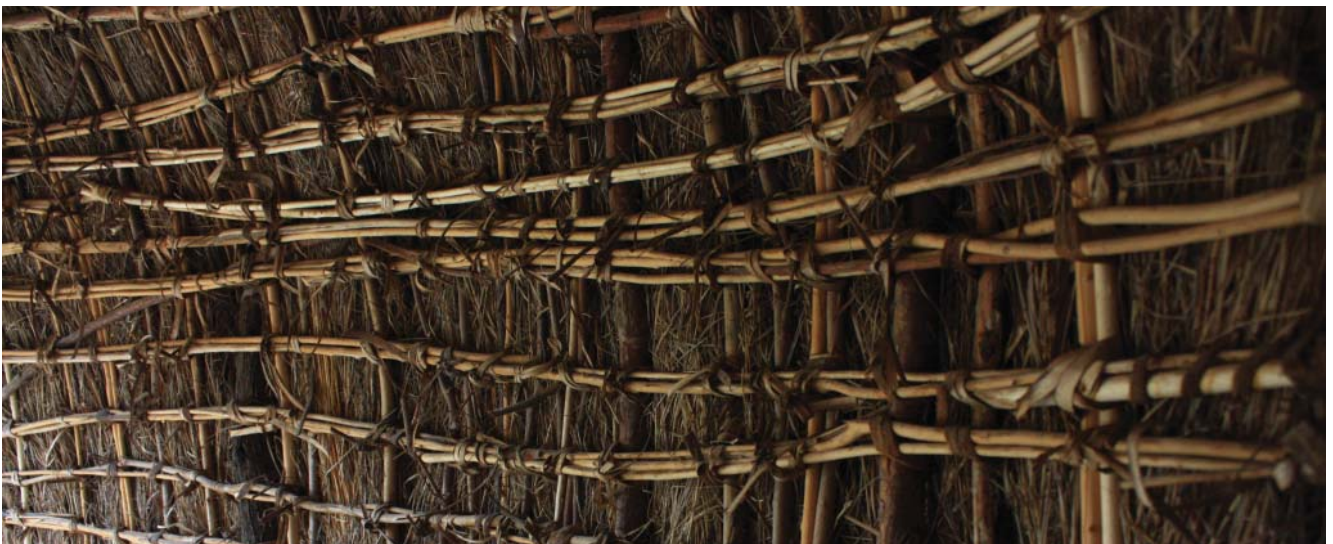
Fig. 293: Awash Fentale woreda: framework of a grass hut consists of vertical members gathered at the crest and horizontal bracing
