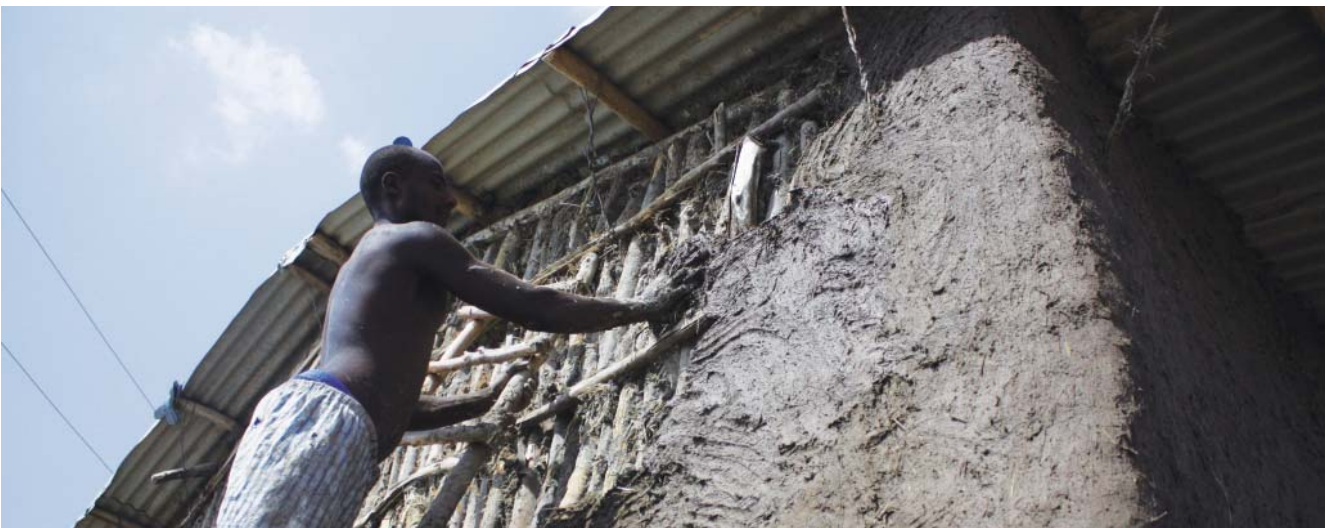
Fig. 154: Logya, Dubti woreda : a Highlander worker plastering wooden structure of a house
