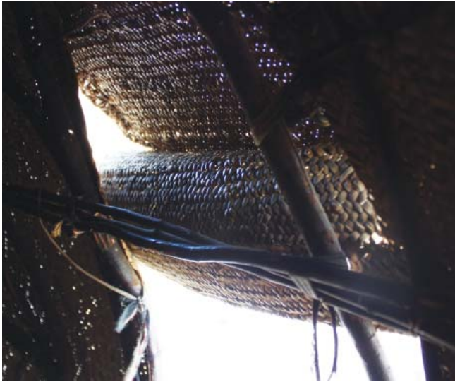
Fig. 243: Logya, Dubti woreda : entrance opening left free in the armature, with pal mat installed above it
