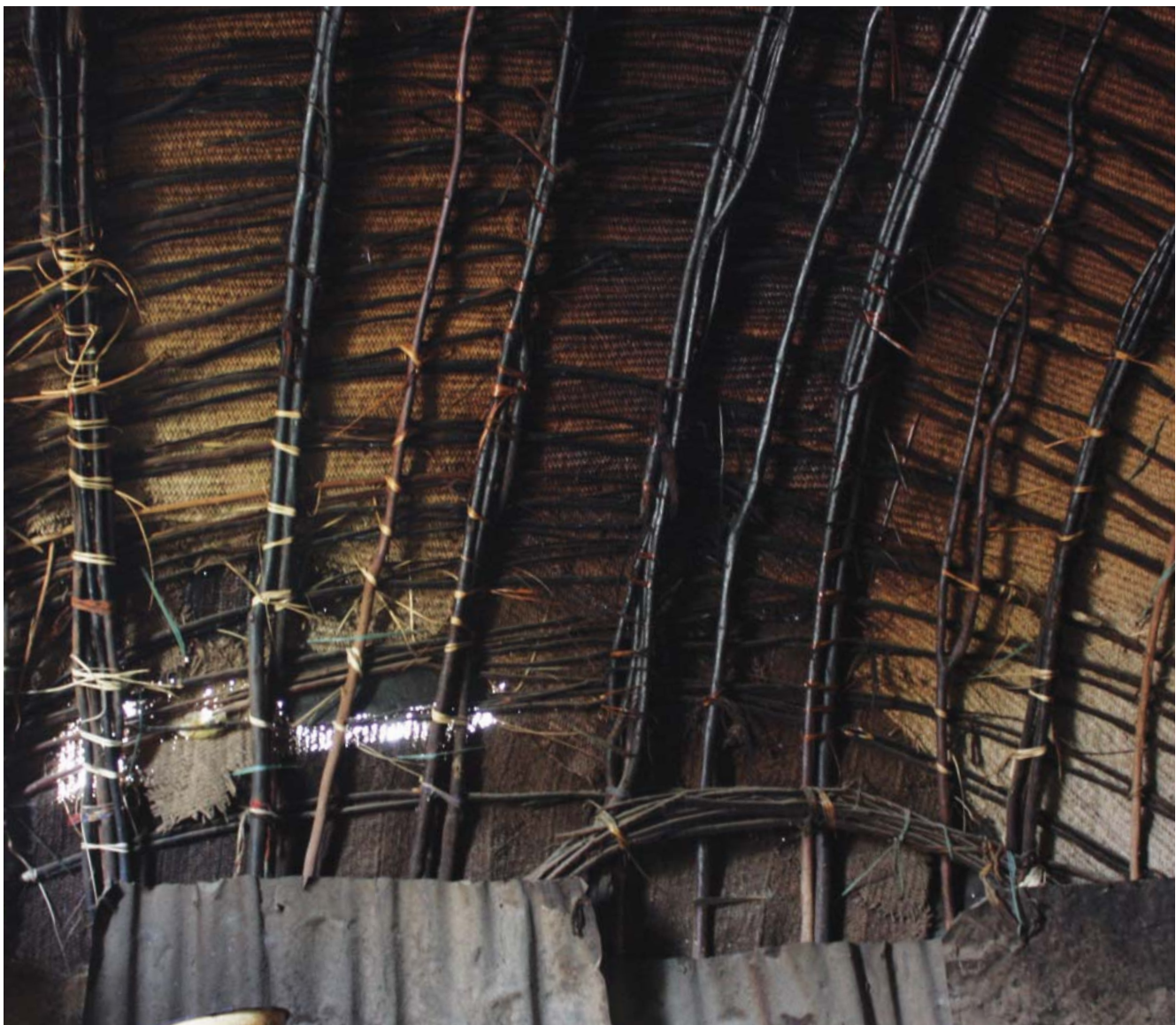
Fig. 231: Logya, Dubti woreda : reinforced rafters halawwa of daboyta armature aligned with the prevailing wind direction in the season
