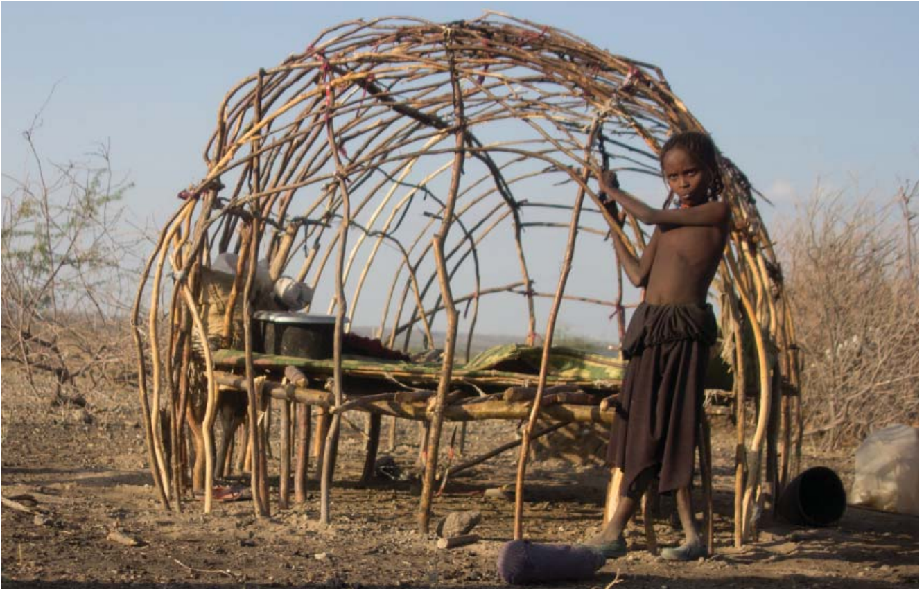
Fig. 260: Frame of an Afar house under construction: a frame is erected around the bed; source: Sebastian Morales 2011 (access 18.12.2016)
