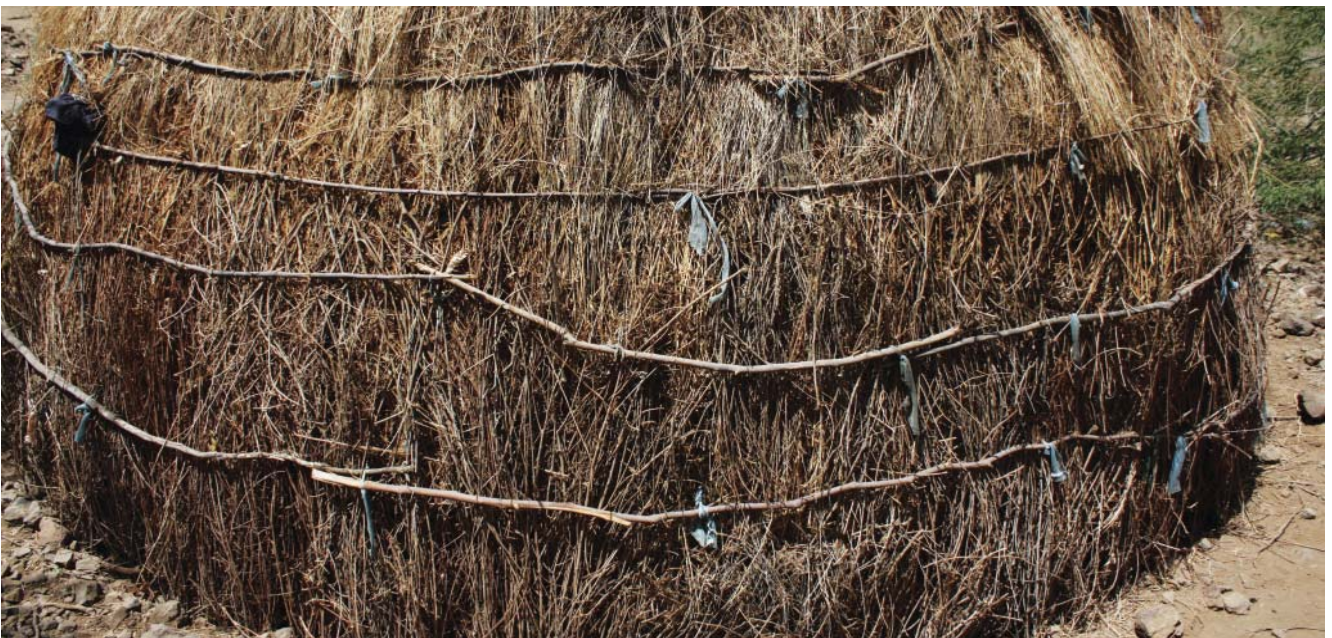
Fig. 304: Gubiyra, Yalo woreda : plain thatch stabilized with split branches, which are tied to the frame and literally clamp the thatch in between
