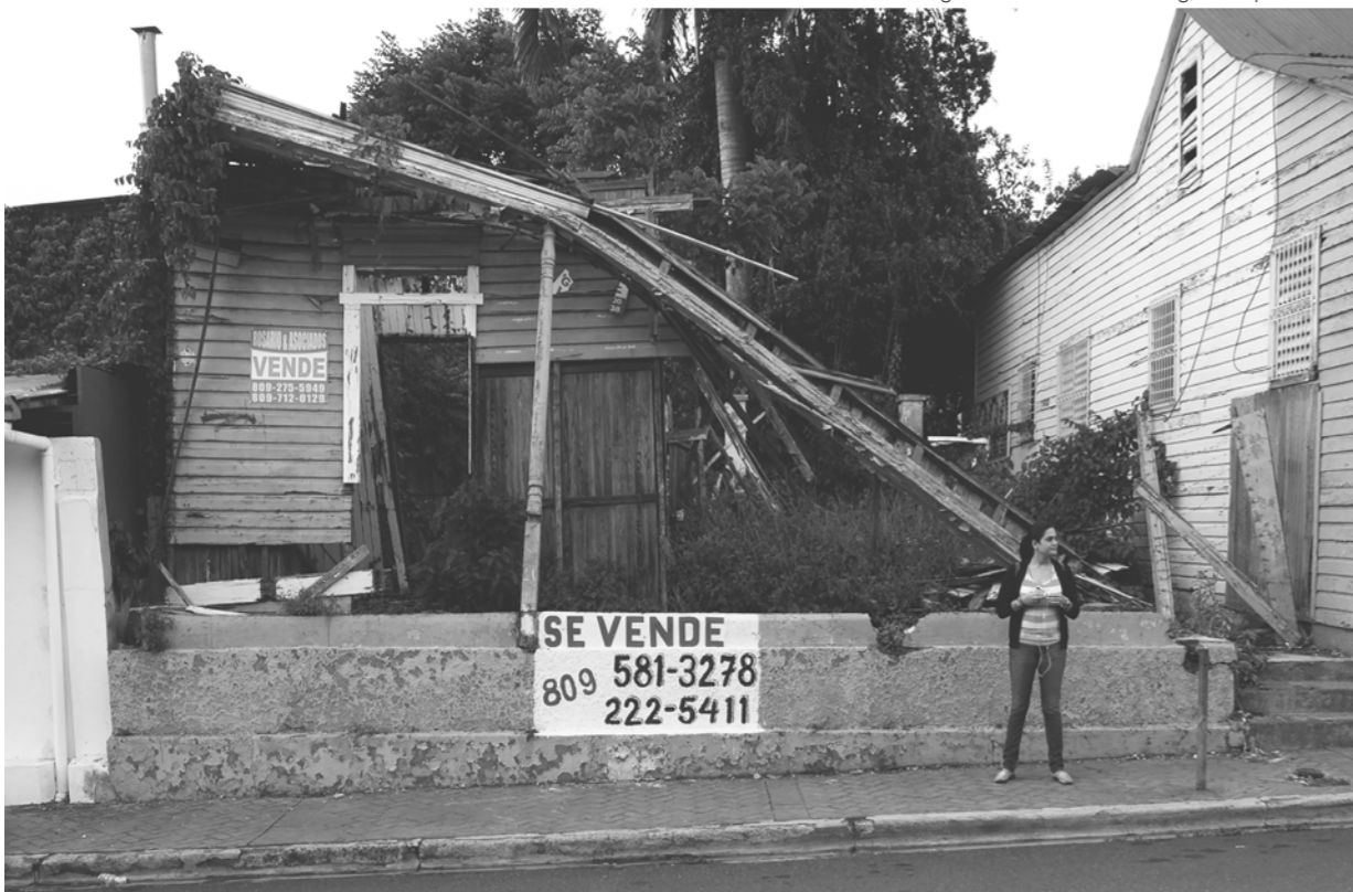
fig.2.25: Deteriorated building, Los Pepines.
