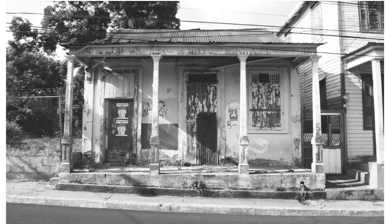
fig.2.29: Lack of knowledge about restoration and preservation of patrimonial buildings, deteriorated wooden house, Los Pepines.
