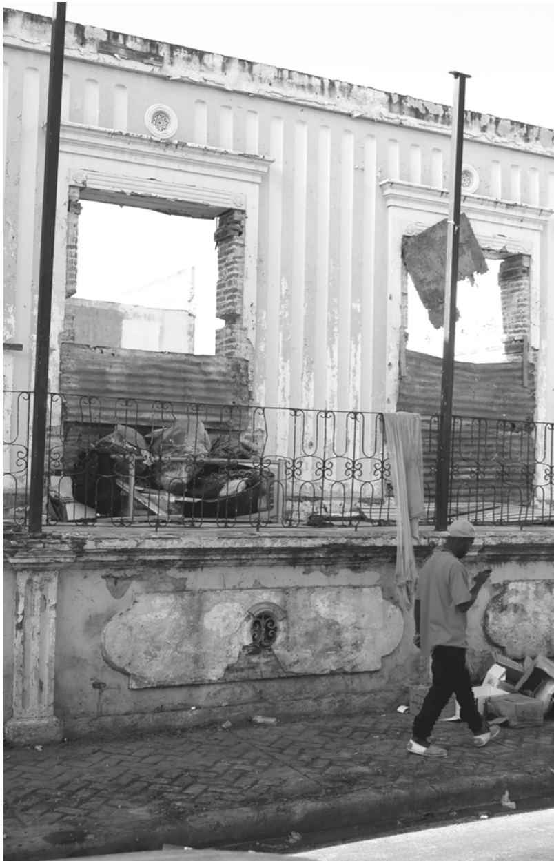
fig.1.7: Patrimonial building falling down. Centro Histórico de Santiago.
