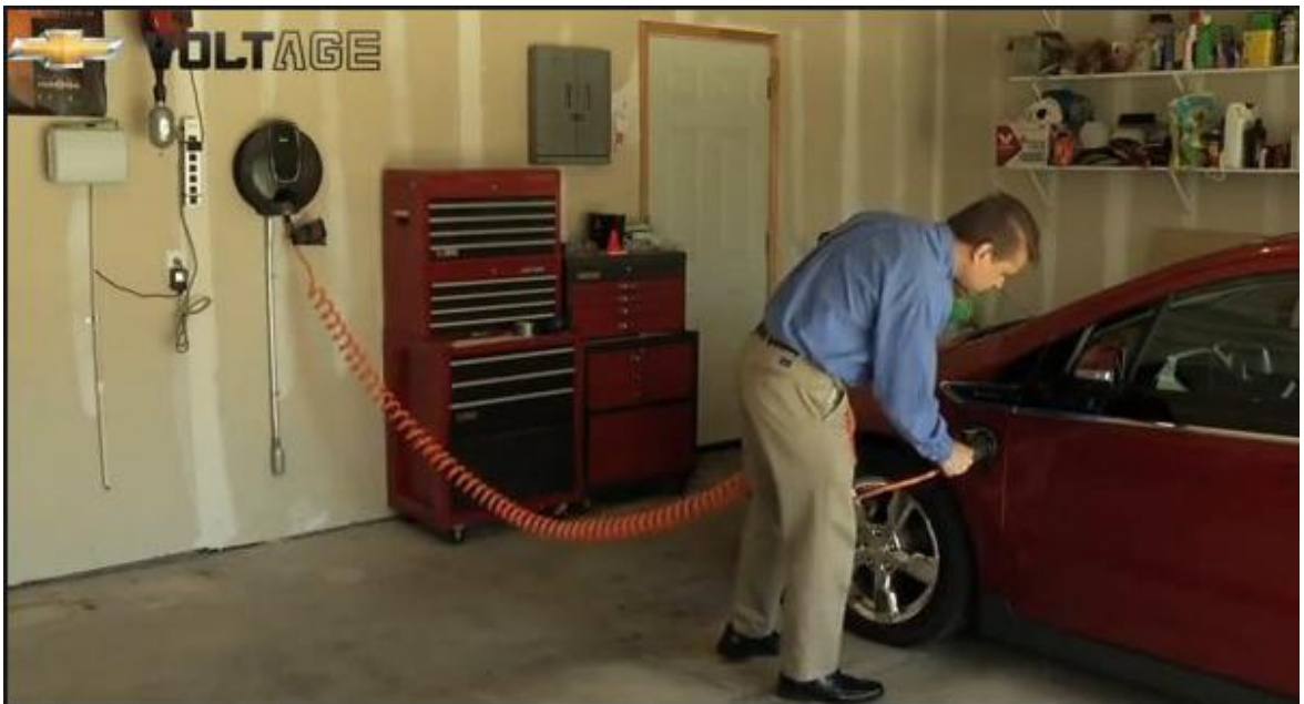
Figure 31: An example of level 2 charging at home using a wall mount (Source: Voelcker, 2017 April 27)
