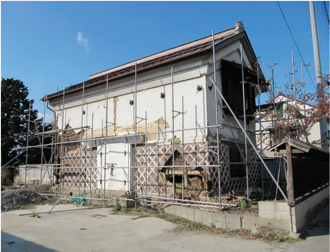
Img. 13: One of many damaged wooden storehouses in Yabuki
