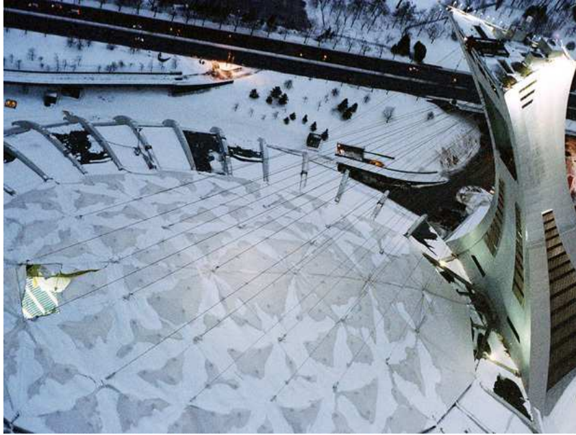
Fig.1 “ Damaged membrane of the Olympic stadium in Montréal under the snow load ”. 1
