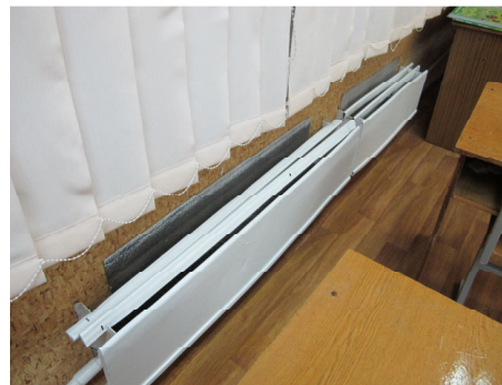
Figure 12: Classrooms convectors. Source: Own
