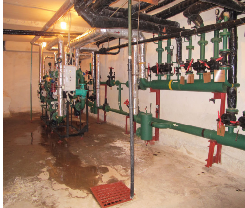
Figure 10: Individual Heating substations in School No 317. Source: Own
