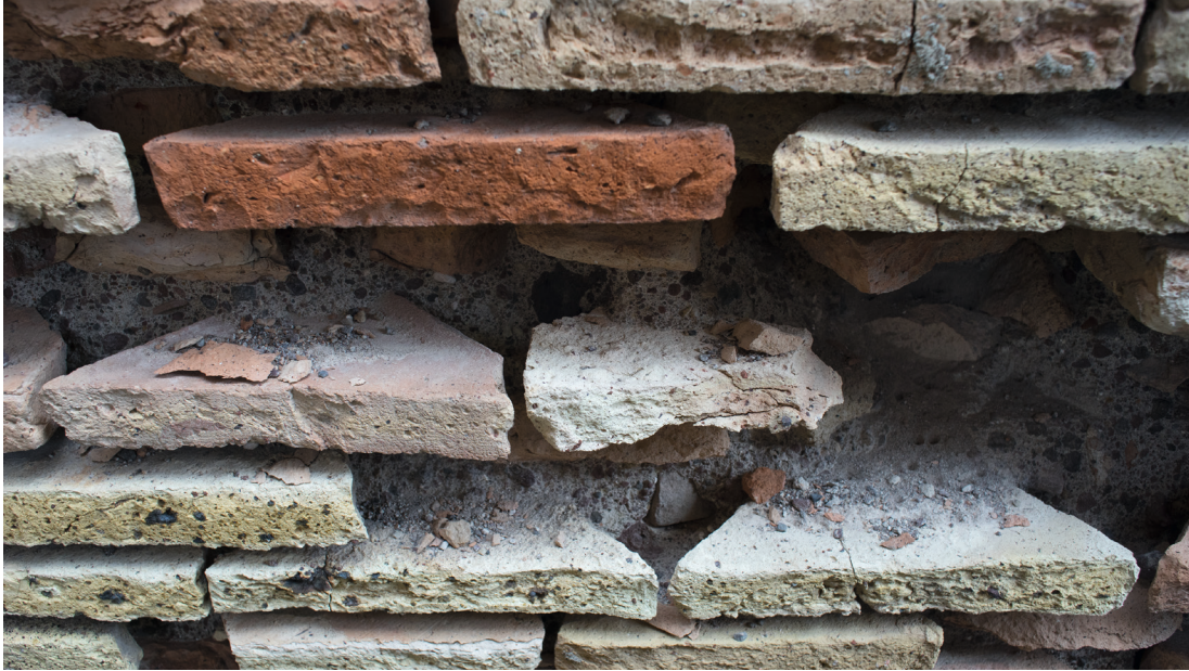
figure 42 - the decay of mortar reveals the triangle shape of bricks in Roman masonry
