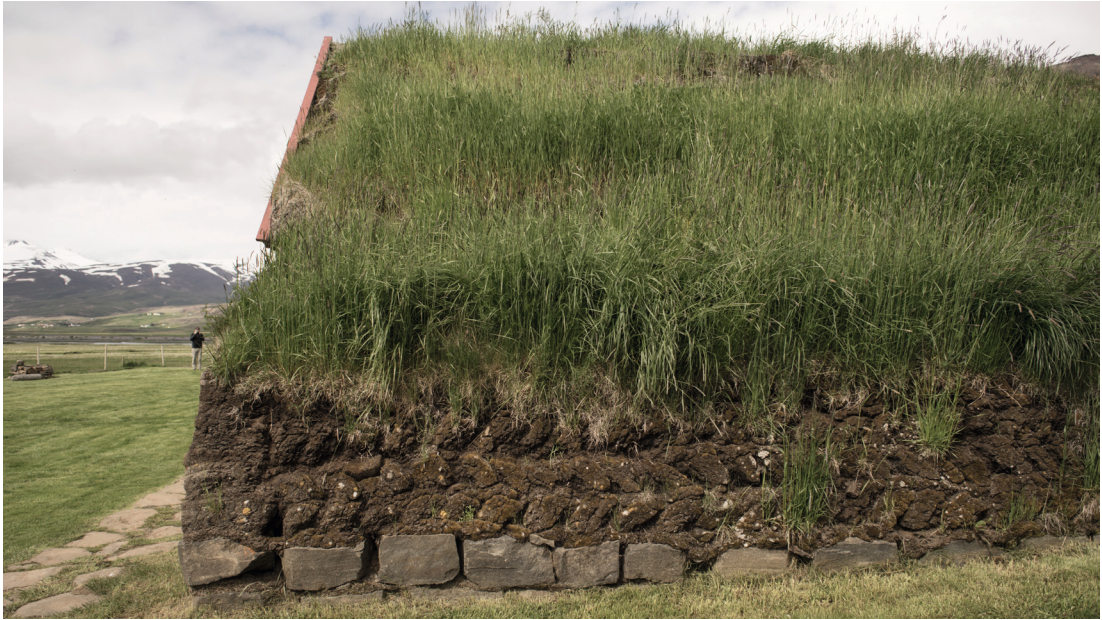
figure 57 - wall being eaten away by decay
