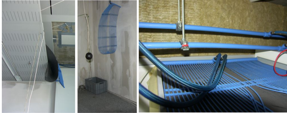
Figure 2.5: Pictures of the cooling ceiling
