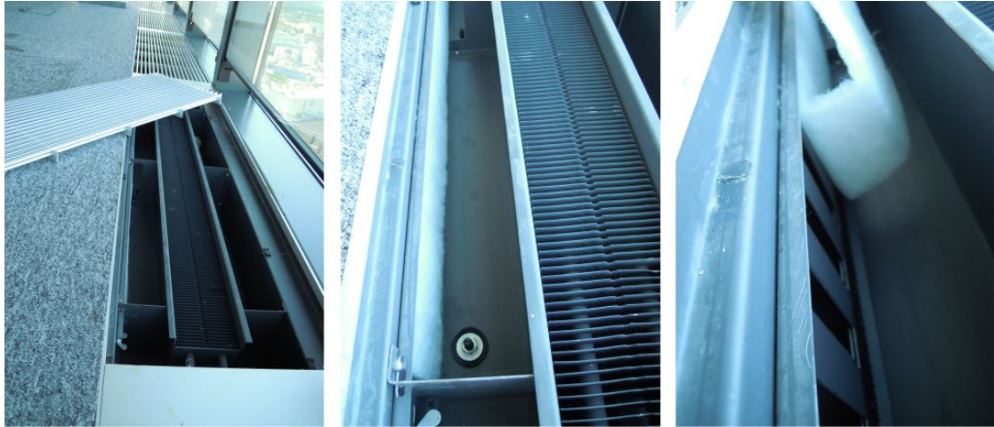
Figure 2.26: Picture of the supply air outlet next to the façade
