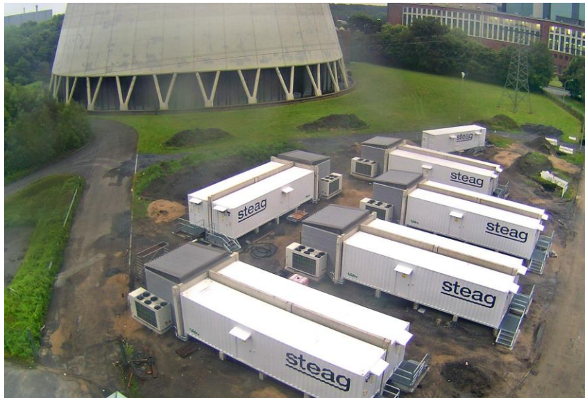
Figure 15: 15 MW power Li-Ion BESS in Lünen [1]
