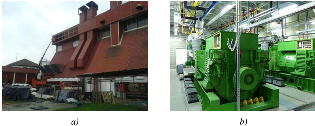
Figure 4: CHP 10 MW plant in the Zapad heating plant, a) view from the outside, b) view from the inside
