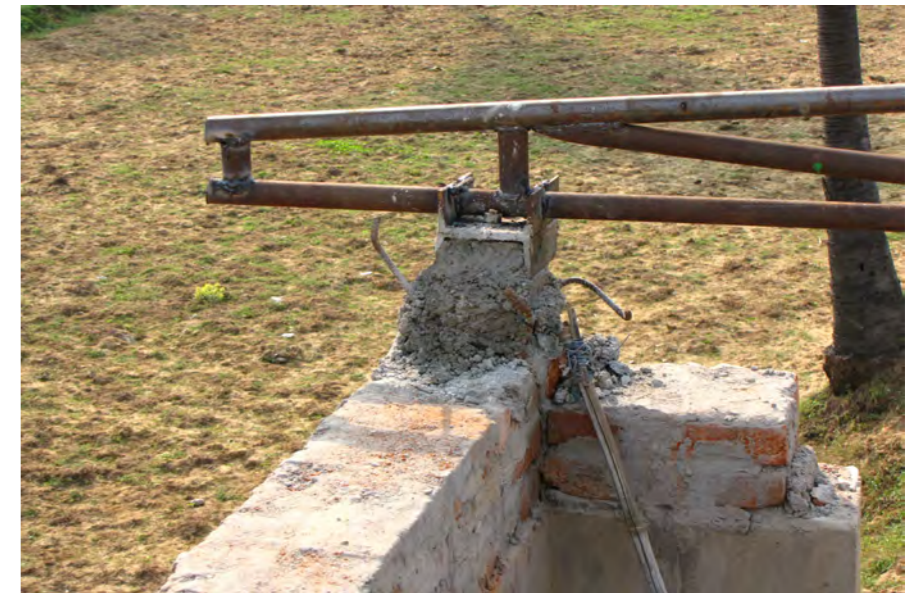
Some works had to be done again
