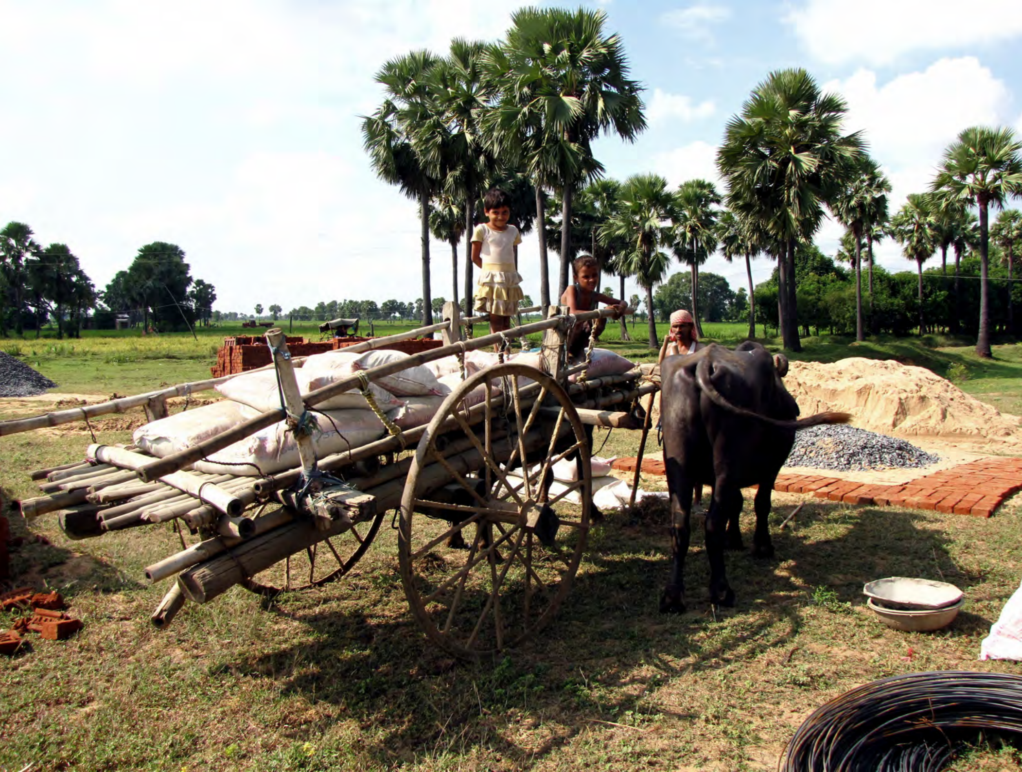
Two water buffaloes bring first delivery of cement to the construction site
