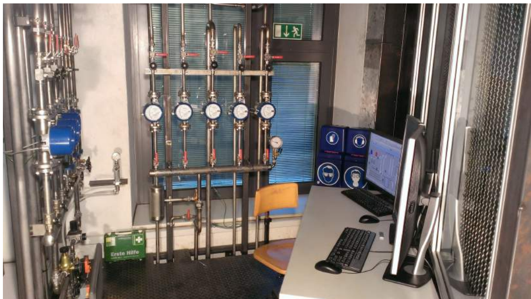
Figure 4.6: Process control system with flow meters for air (left), steam (middle), and computers to operate the PCS (right)
