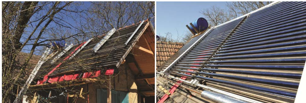
Figure 19: Solar collector (vacuum type) on the roof of the energy-autonomous house model
