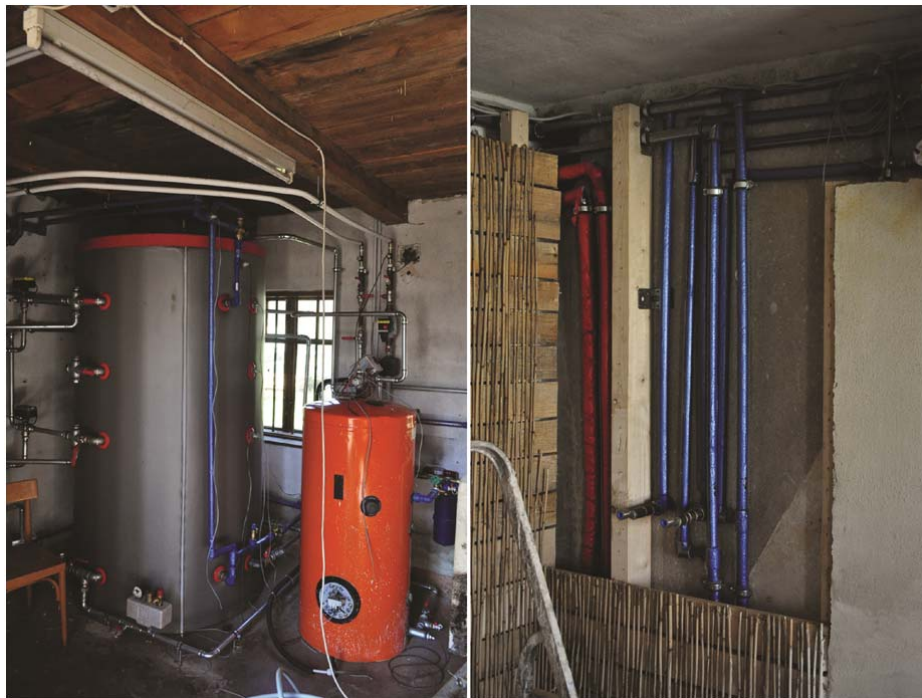
Figure 20: shows the hot water storage and piping system in the energy-autonomous house model
