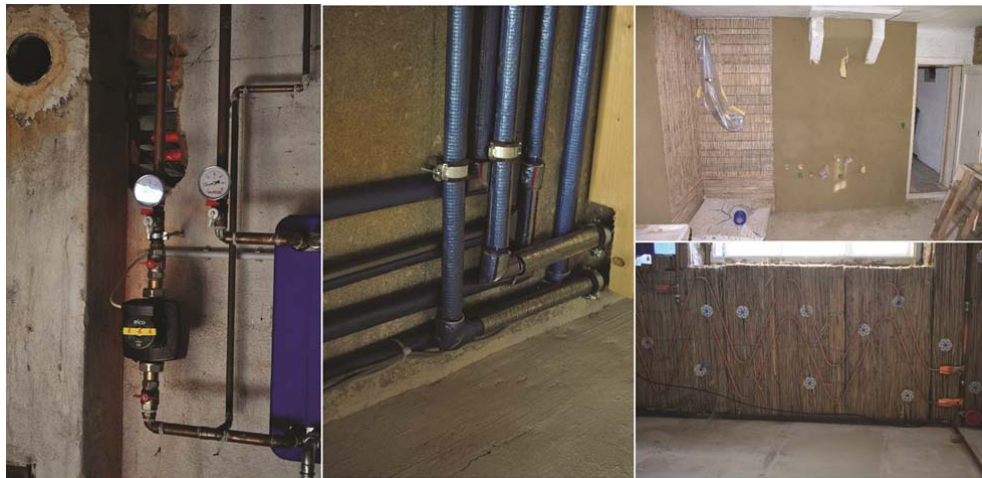
Figure 17: Hot water piping system in the energy-autonomous house model
