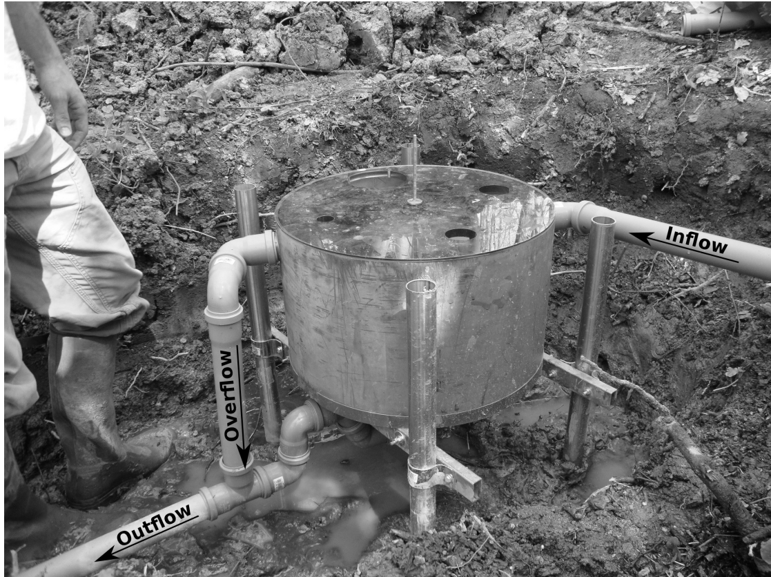
Figure 2.2: Fully assembled and installed WME with foundation poles. The holes in the lid of the WME are for the placement of the measurement sensors.
