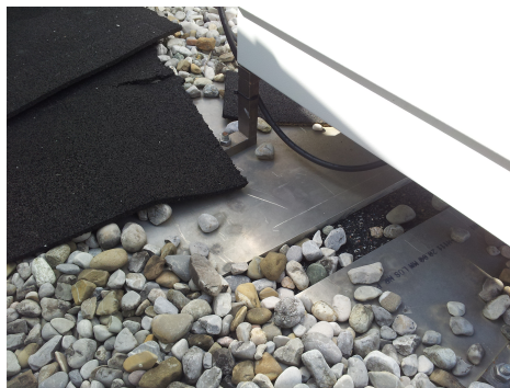
Figure 4.4: Rack standing on alloy plates laying on the rubber layer of the roof.
