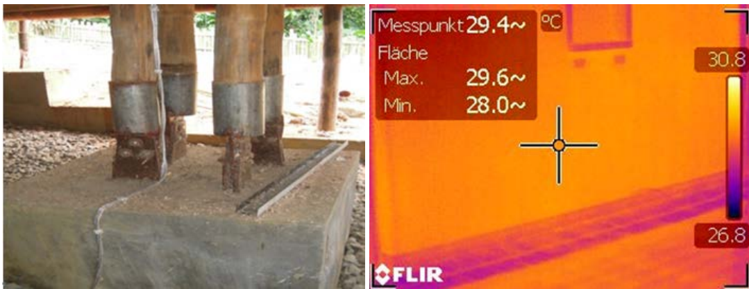
Figure 8: Point foundations with steel joints; thermographic photo of ventilation slots
