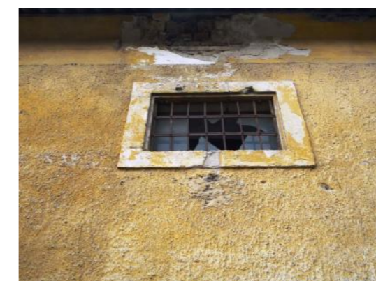
Abb. 57 Zerbrochenes Fenster (Ost)
