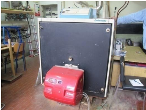
Figure 14 the ELFO boiler for heating
