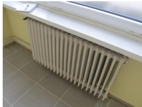
Figure 15 Installed radiator types at school
