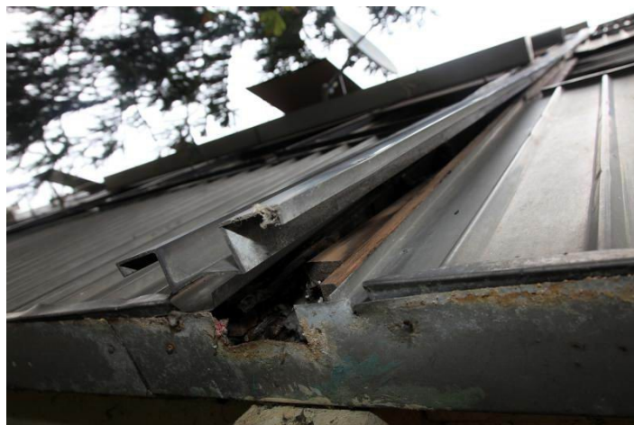
Figure 10 Damages of the metal coverings (Photo collection of the author)
