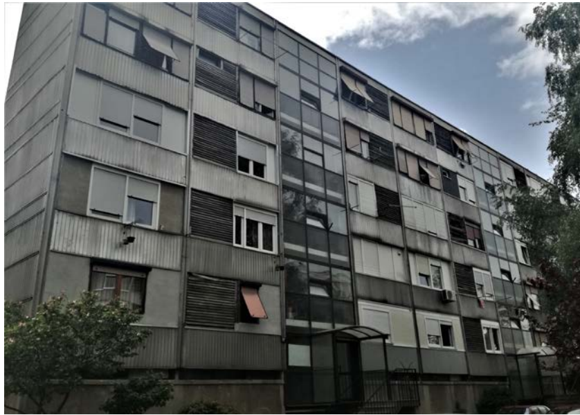
Figure 8 Current state of the front façade (Photo collection of the author)
