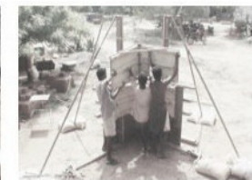
Lifting panels of the first form to the third one of a corner wall
