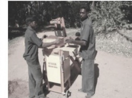
Handling the block to stack it near the press for the initial curing
