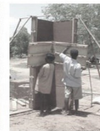
Lifting panels of the second form to the fourth one of a corner wall
