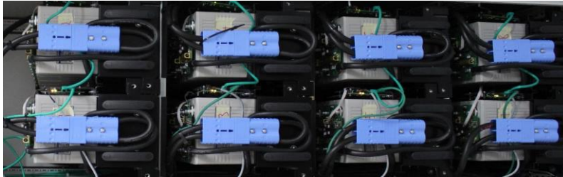
Figure 6-14 LiFePO 4 Battery Packs of the ESS at the WEB Microgrid (own picture)
