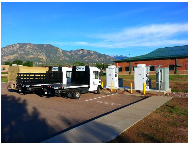
Figure 5-4 Bidirectional Charging Station for Electric 73
