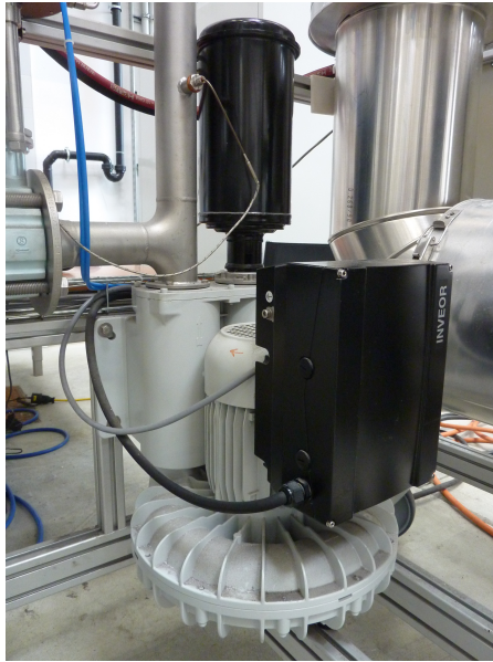
Figure 4.5: Elektror Compressor with frequency converter and filter
