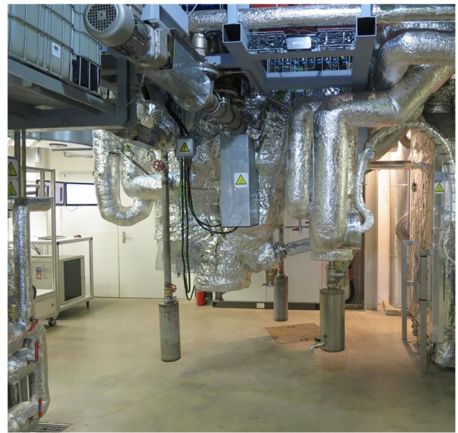
Fig. 7 Picture of the pilot plant with thermal insulation and ash containers (lower floor)
