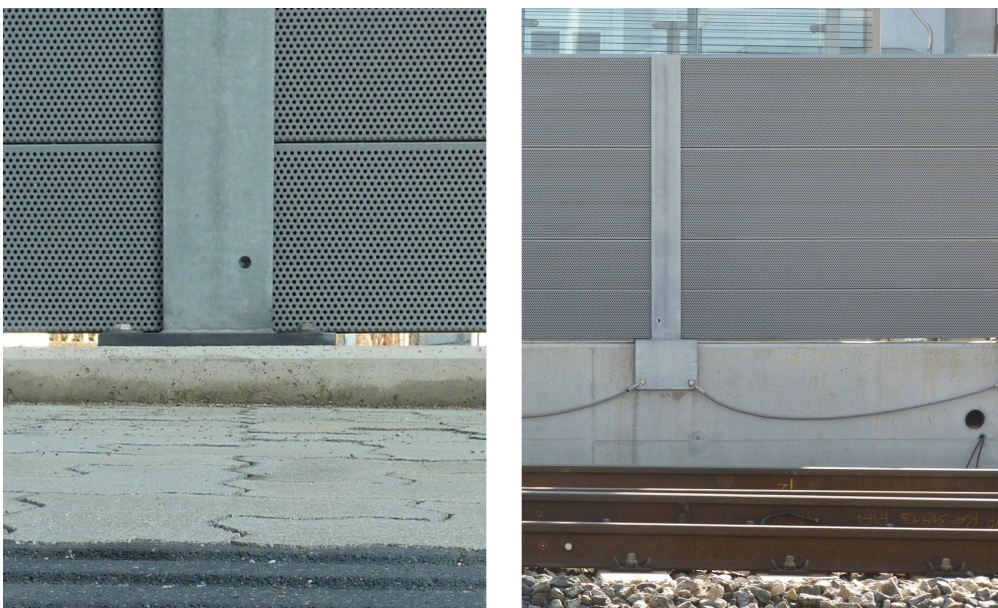
Figure 1.3: Gap underneath a noise barrier
