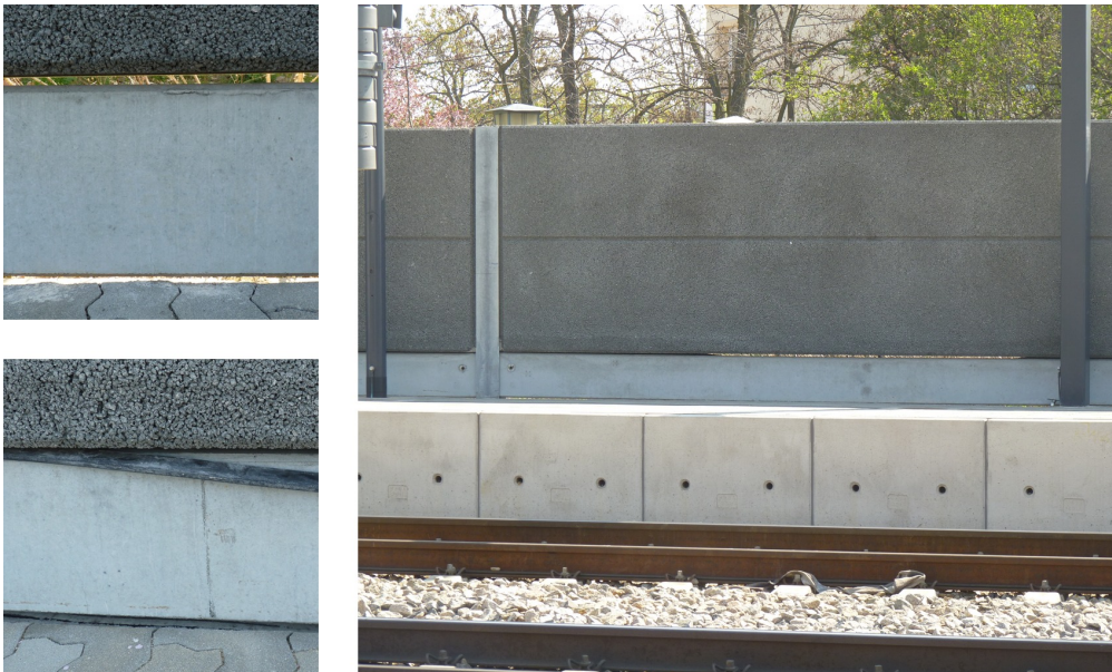
Figure 1.2: Gap between noise barrier elements
