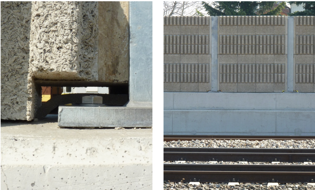
Figure 1.4: Holes around the base of the post
