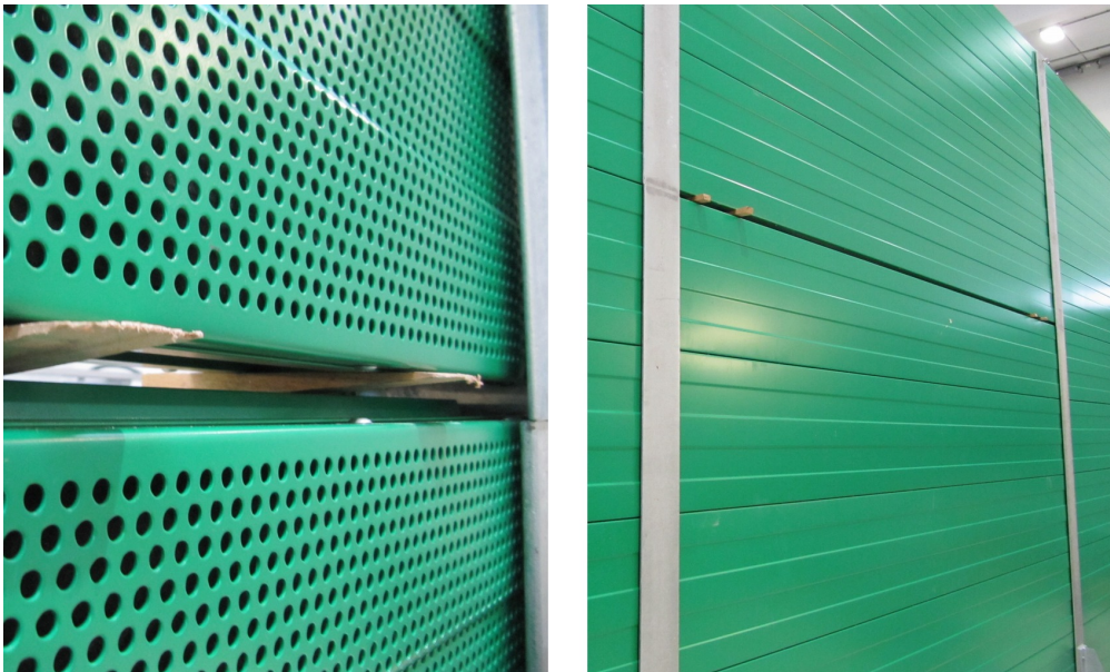
Figure 3.1: The noise barrier where the measurements have been carried out. The gap shown is the largest one that has been examined (2 cm)
