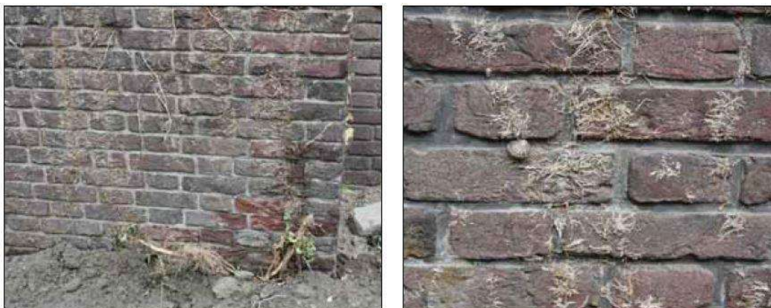
Figure 6 : Picture of façade damage caused by self climbing plants (Source: GREENSCREEN 2017 )
