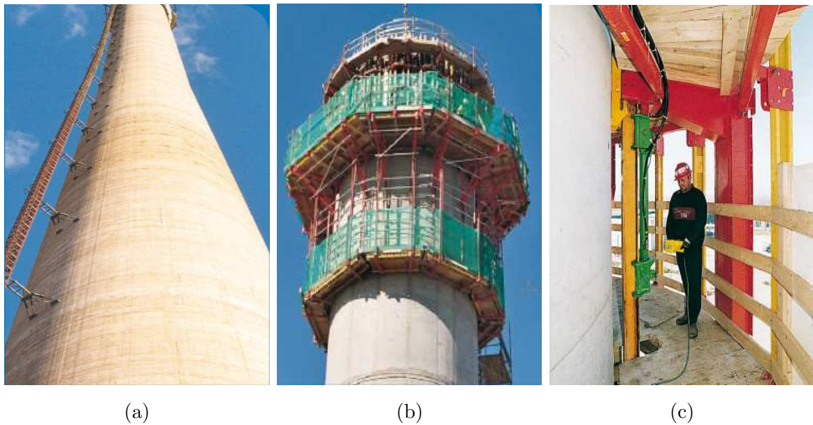
Figure 2.10: In-situ slip form method, taken from [17]; (a) concrete tower; (b) slip formwork; and (c) working platform in slip formwork
