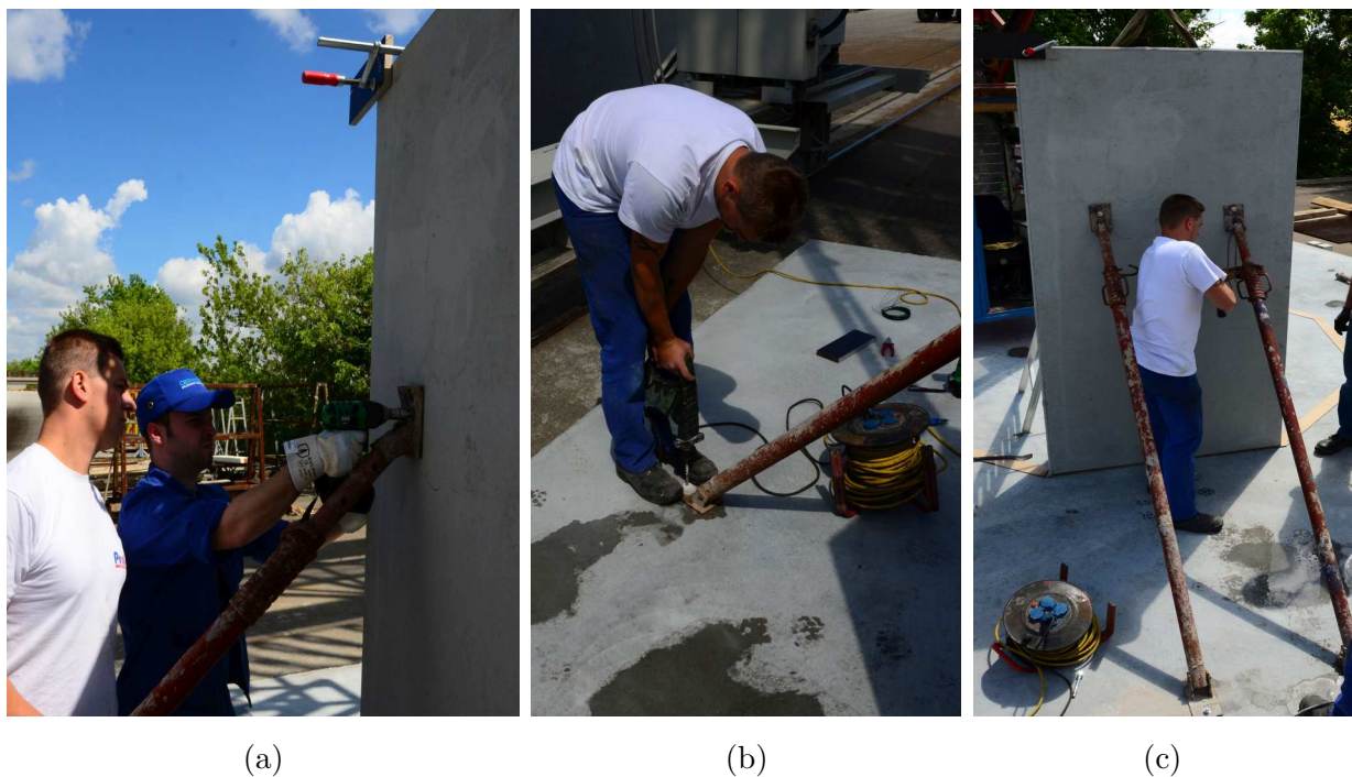
Figure 4.56: Installation of the screw bracings; (a) into the element; (b) into the foundation; and (c) placed bracings
