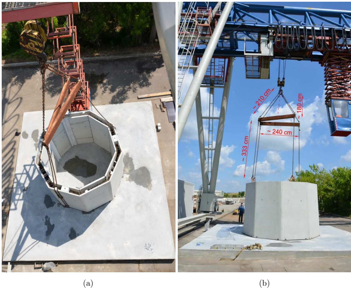
Figure 4.73: Lifting set up; (a) top view of the segment with lifting set up; and (b) side view of the segment with lifting set up
