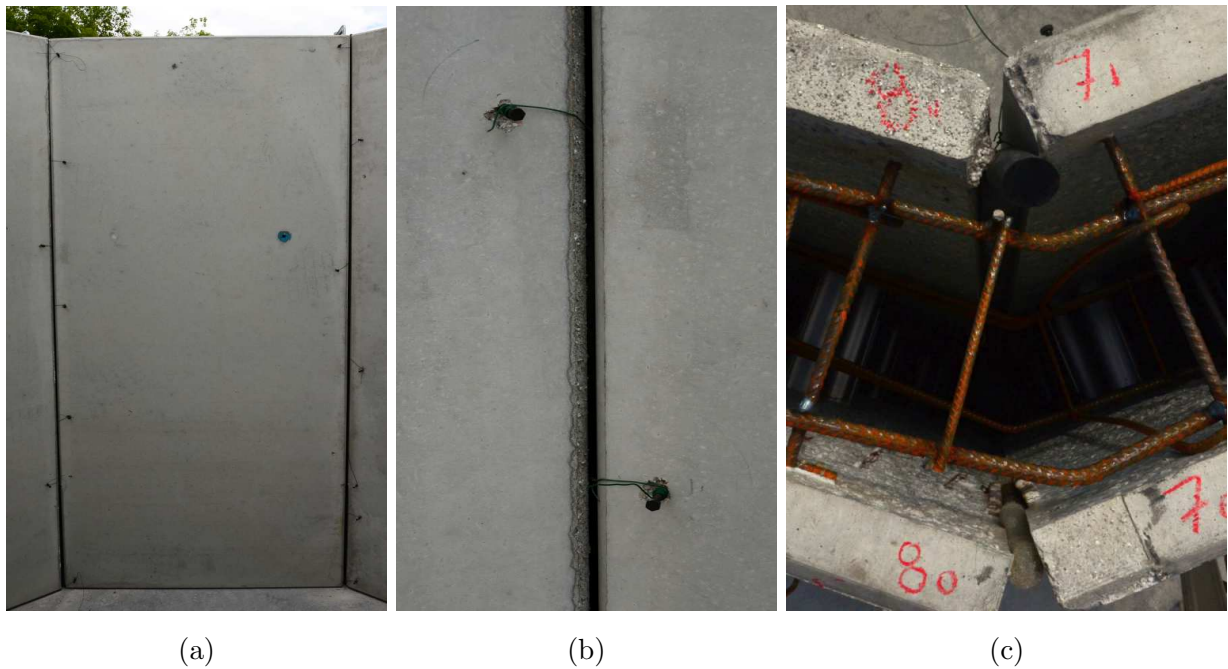
Figure 4.67: Vertical joints with embedded EPDM tubes; (a) installed tubes; (b) wires tied to screws; and (c) top view
