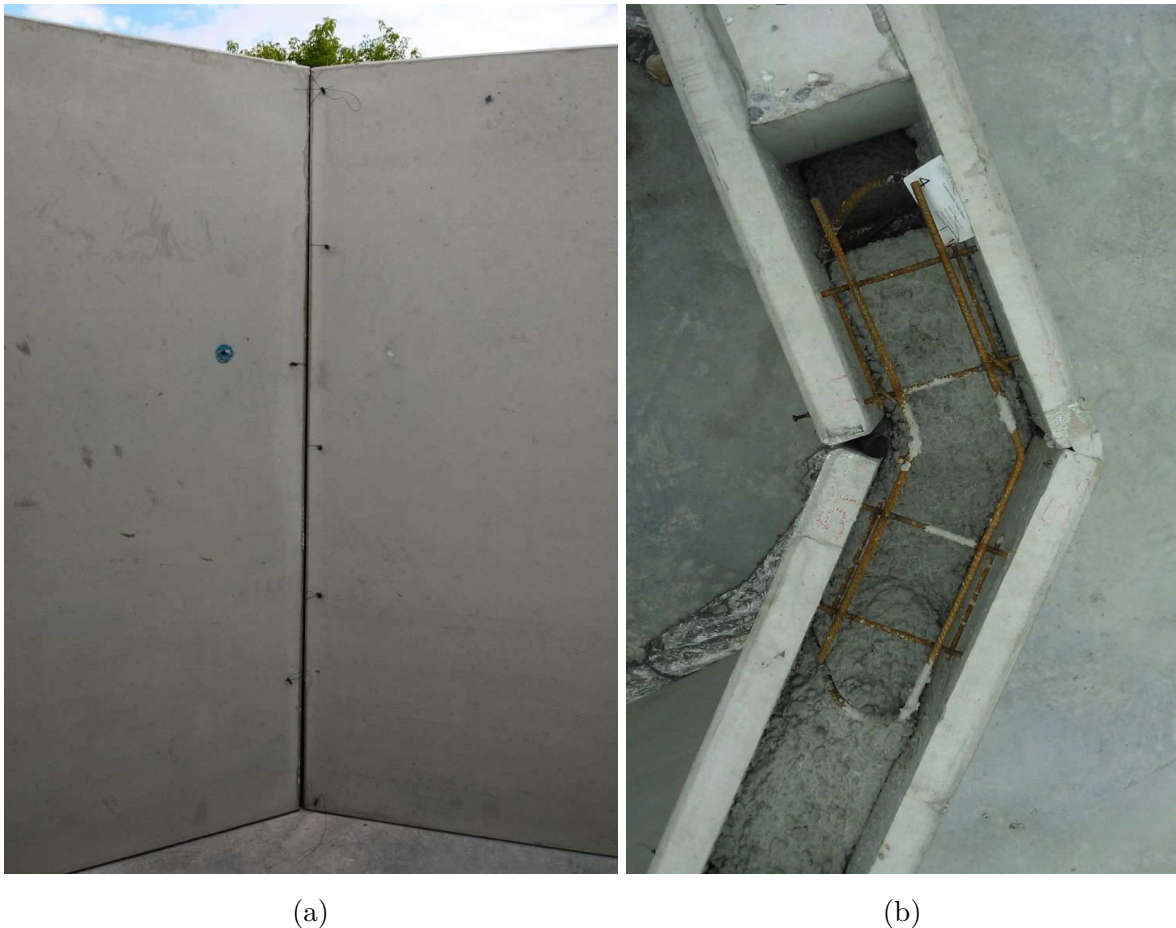
Figure 5.11: Inner vertical joint sealed by elastomer tube; (a) view from inside; and (b) top view
