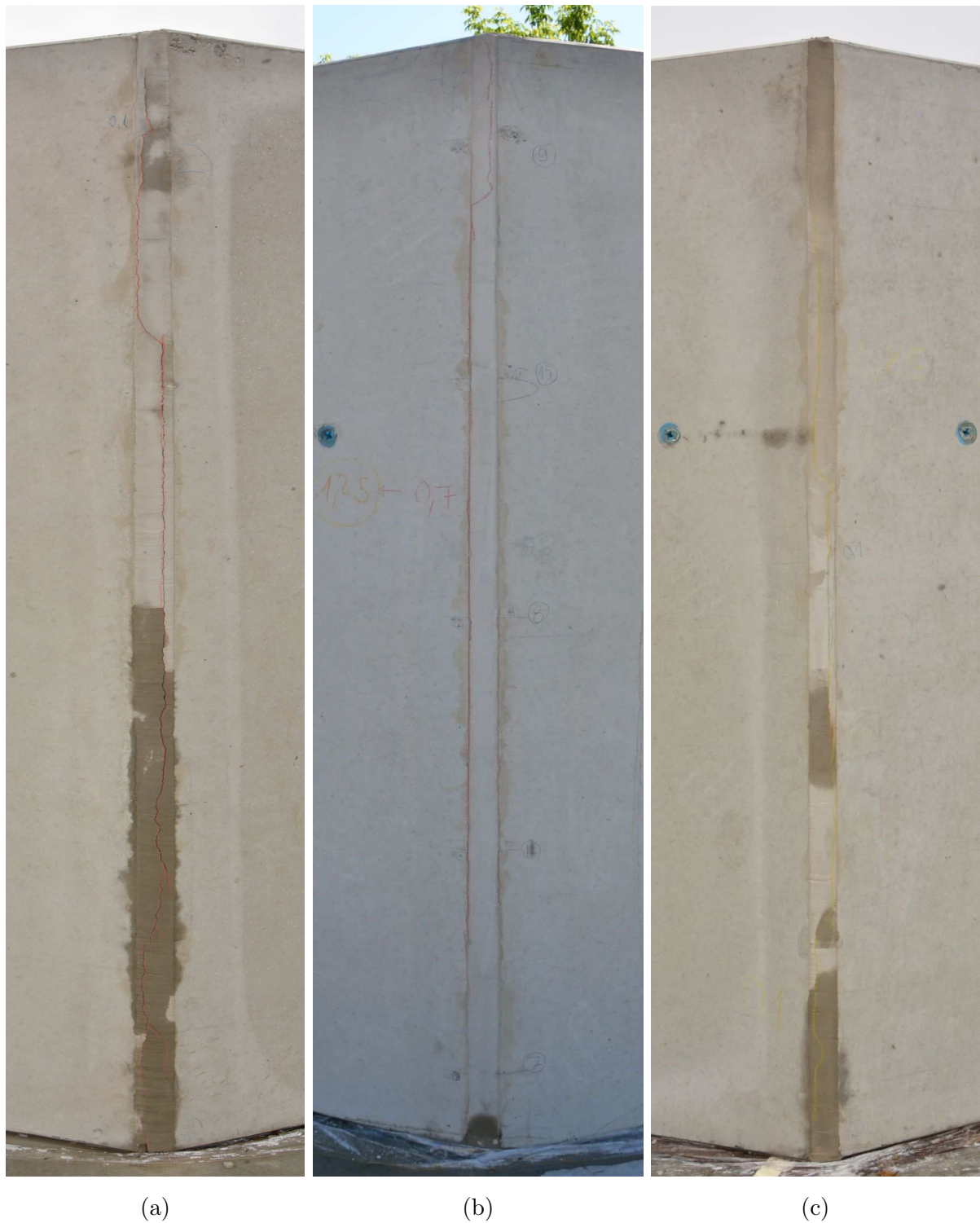
Figure 5.14: Cracks pattern for different edges surfaces of outer shell; (a) type R-R: joint between elements 3-2; (b) type S-R: joint between elements 4-3; and (c) type S-S: joint between elements 6-5
