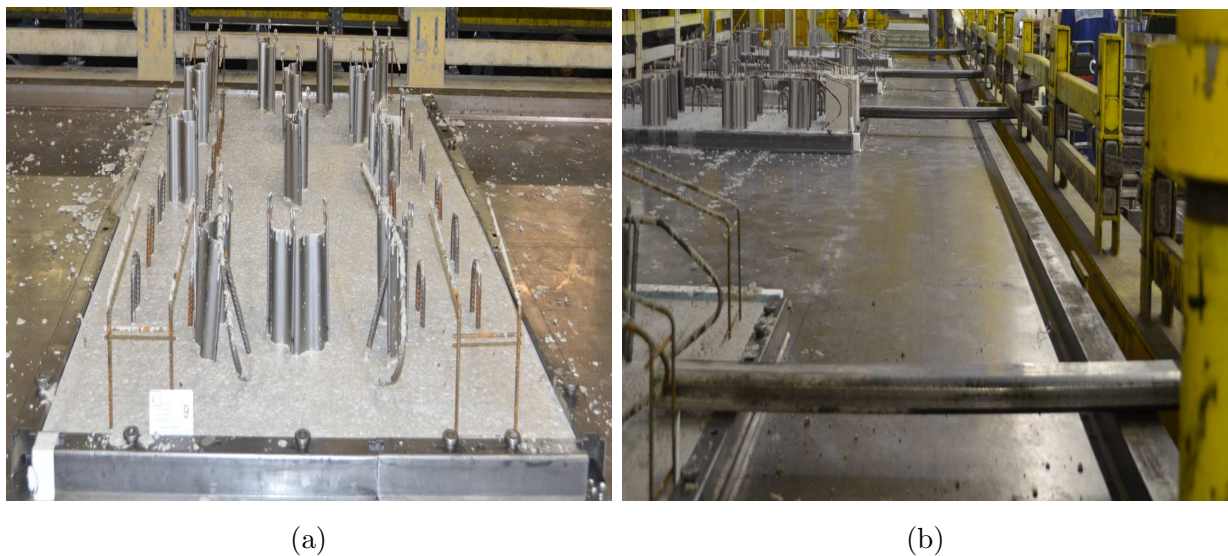
Figure 4.40: Fixing of the first shell in the turning device; (a) hardened concrete shell; and (b) concrete shells fixed in turning device by steel arms
