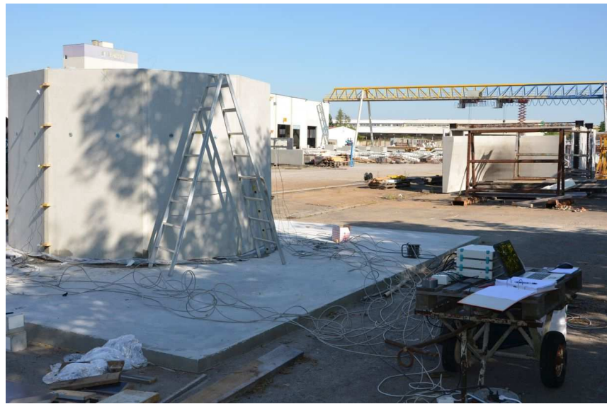
Figure 5.18: Installed and connected measuring equipment
