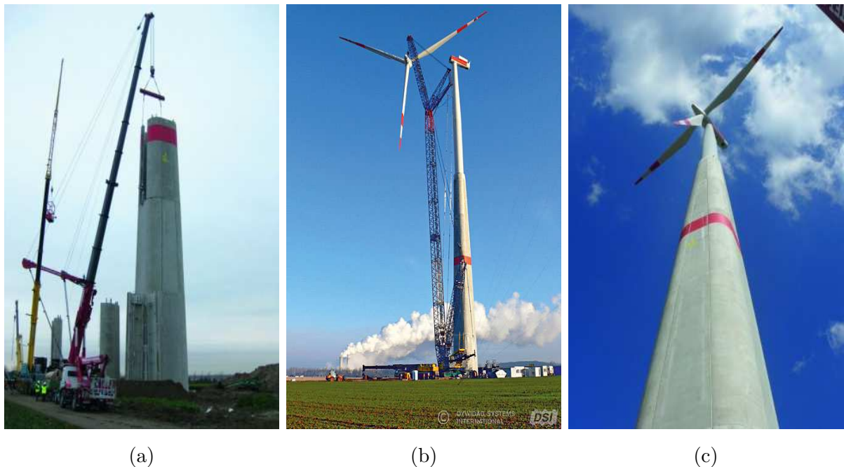
Figure 2.16: ATS wind tower during construction, taken from [18]; (a) assembling process; (b) placing of the nacelle; and (c) assembled tower
