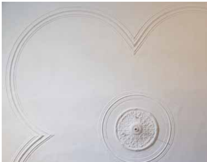
Abb.126: Stuckdecke in OG_03 (Türk, 30.03.2018)
