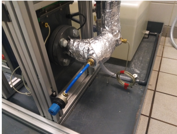
Figure 3.3.: Safety valve and temperature sensor (PT100) after heater
