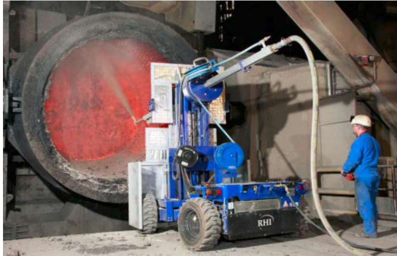
Figure 1.1.2: Manual gunning maintenance of a ladle. The gunning manipulator is remote controlled by the steel worker. The machine needs a heat shield, because the empty ladle is still extremely hot [96].
