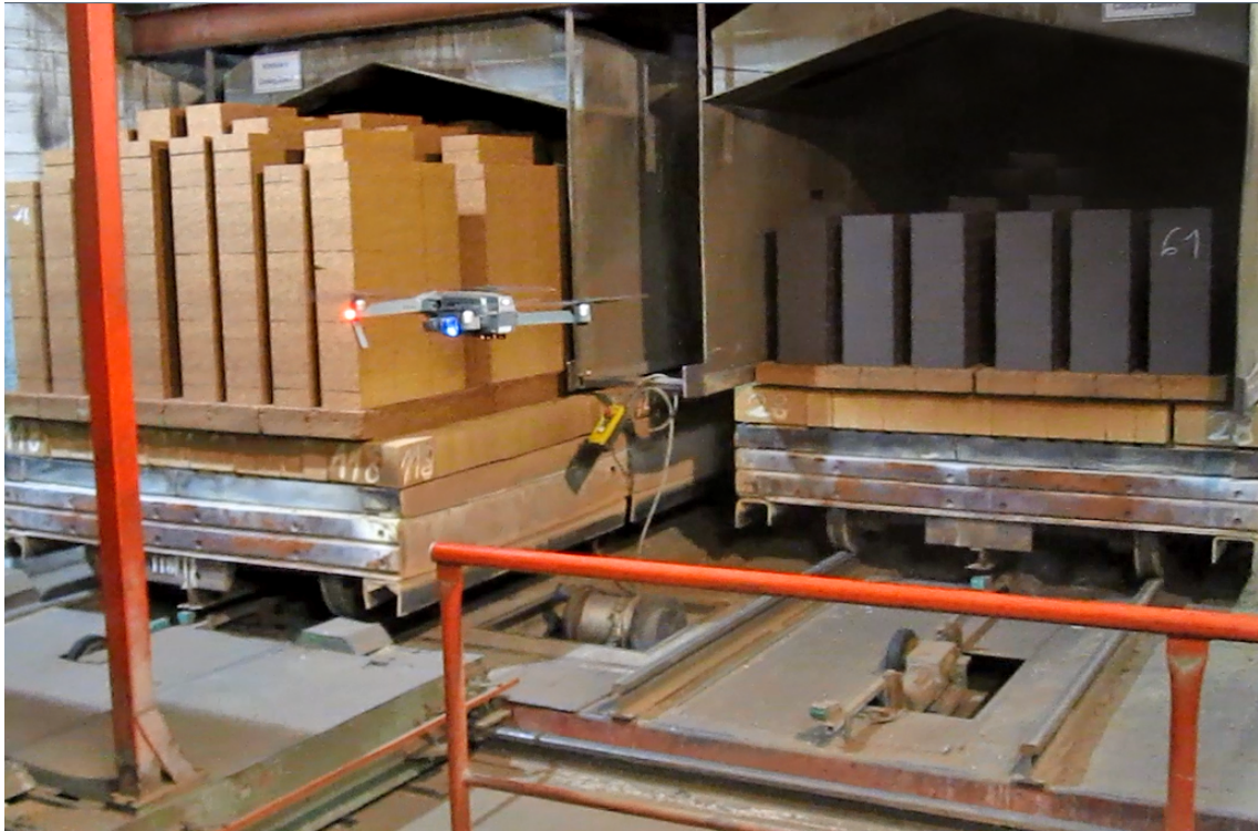
Figure 3.3.6: Area at the end of the tunnel kiln. The pentagonal tunnels in the background are blowers to cool down refractory.
