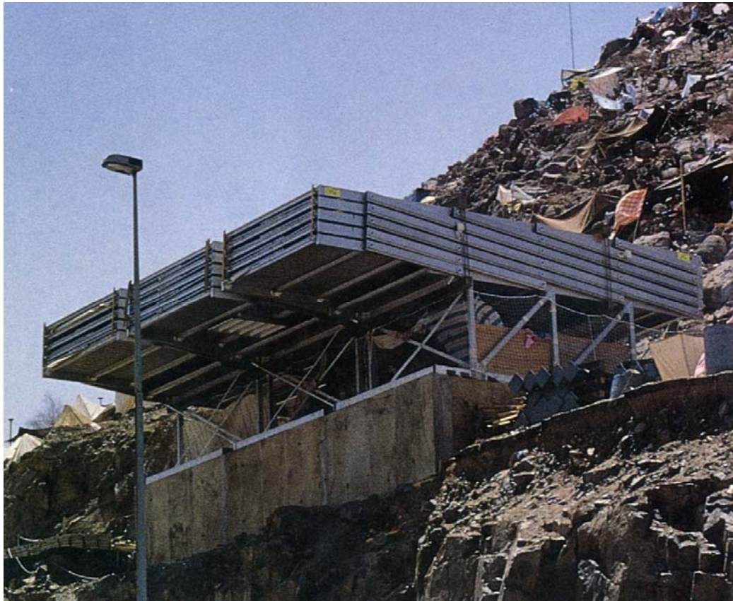
Figure 4.12 The prototype installed on top of a hill side podium to exemplify its versatility and adaptability to the mountain terrain.
