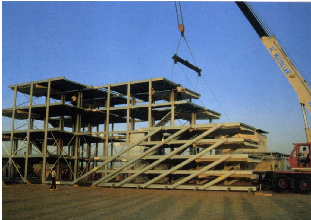
Figure 4.11 The foldable structure being erected near the Hajj Research Centre in Jeddah for testing and demonstration.
