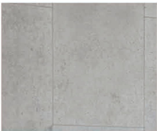
Interior wall cladding (VeroStone, Jura Cream)
