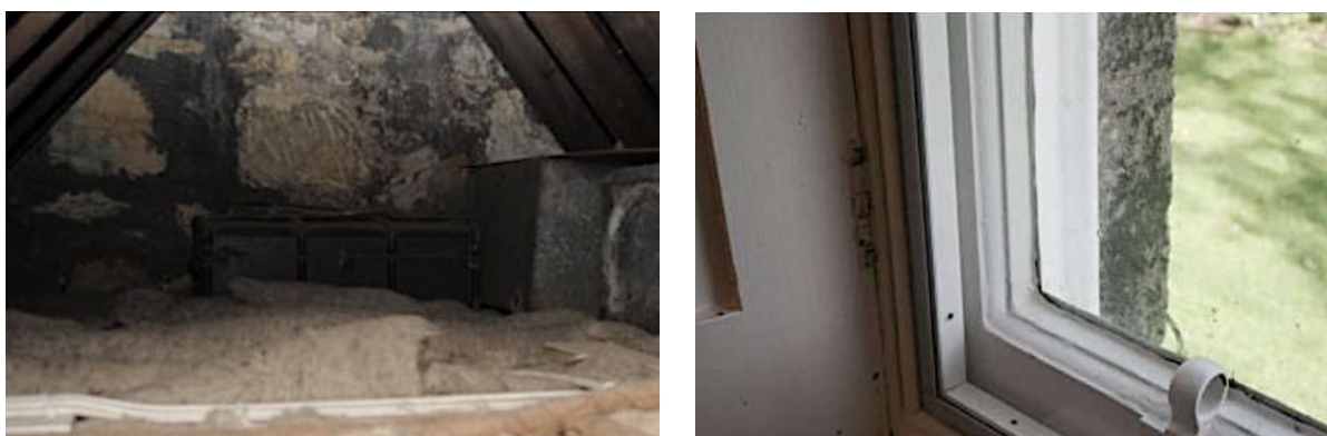
Fig. 51 Left: Sheep's wool insulation, right: Polycarbonate secondary glazing in place (Historic Scotland, 2012, p.9)
