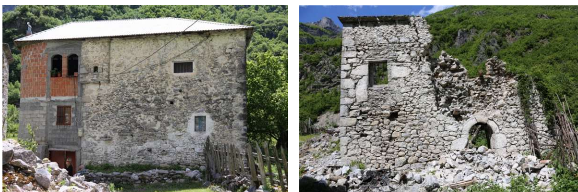
Fig. 33 Left: Inadequate interventions in kulla, right: Damaged kulla, Valbona, 2021
