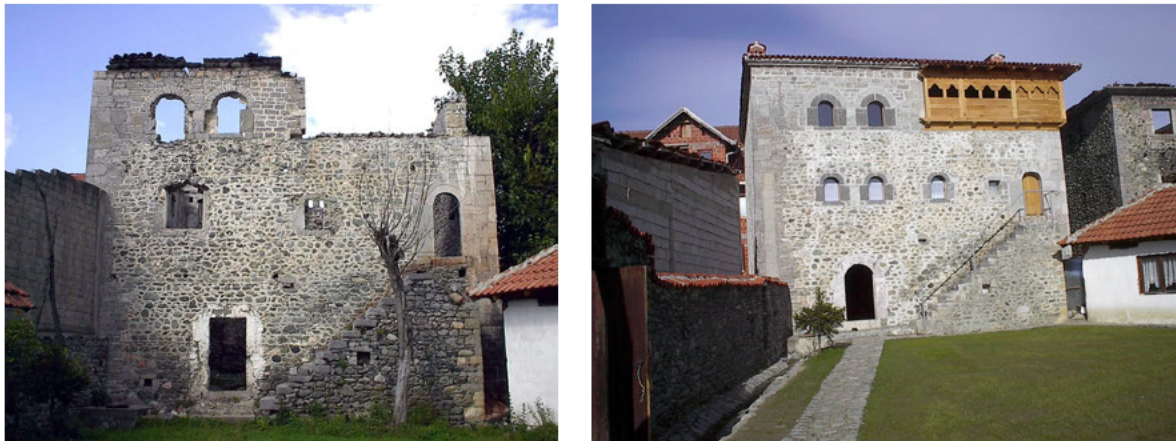
Fig. 35 Reconstruction and adaptive reuse of the Kulla Oda e Junikut during 2001-2002 as a library; Left: before intervention (CHwB Kosova, 2001), right: after intervention (CHwB Kosova, 2019)
