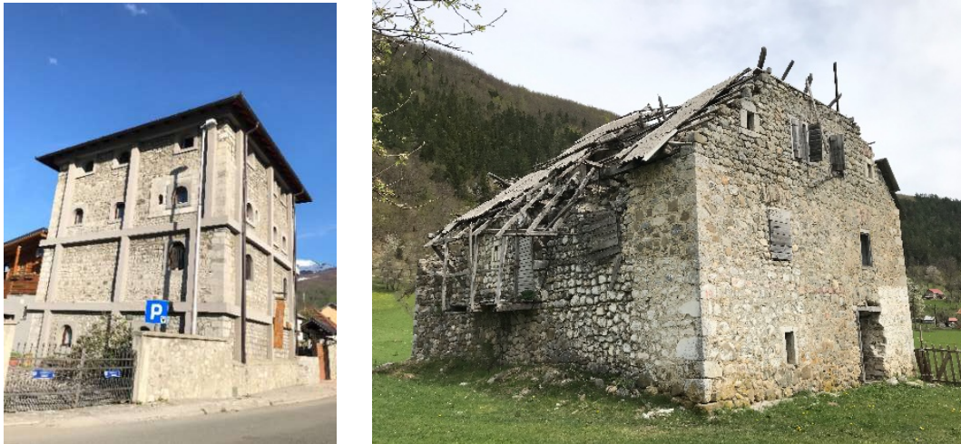
Fig. 32 Left: Inadequate interventions in kulla, right: Damaged kulla, Guci (Labeatët, 2021)
