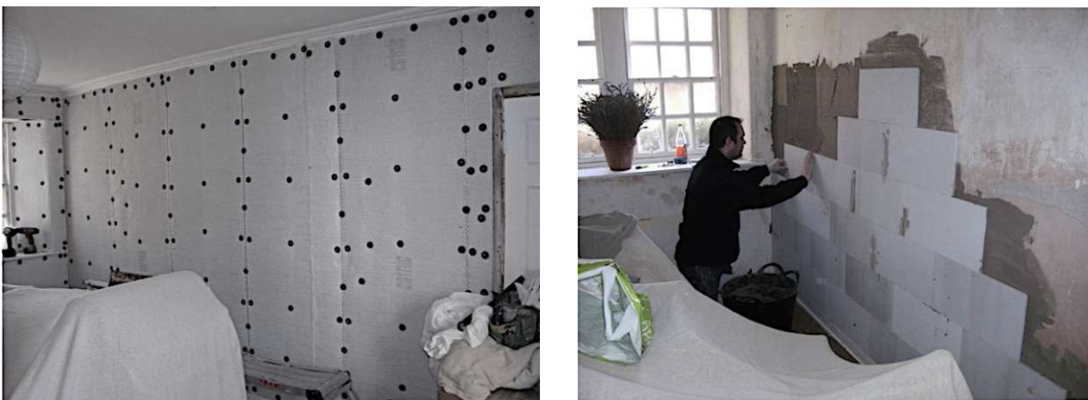
Fig. 56 Left: Aerogel insulation before applying the plaster finish, right: Calcium silicate board being applied to the masonry wall (Historic Scotland, 2012 b, p.5-10)
