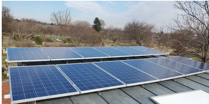
Figure 3.1: PV test site with the twelve coated modules mounted on the roof.
