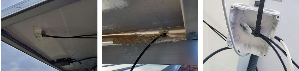
(a) Sensor 4 mounted on the corner of Module 1 (Remsolar). (b) Sensor 1 mounted on the corner of Module 7 (Dowsil). (c) Sensor 5 measuring the ambient temperature.
