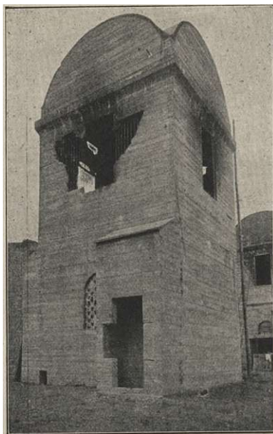
(b) South-west side of the building after the fire on the first floor
