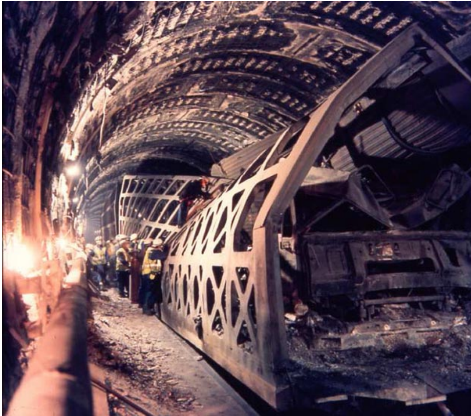
Fig. 2.5: Damage to the concrete lining of Channel tunnel after the fire in 1996 (picture by Eurotunnel)
