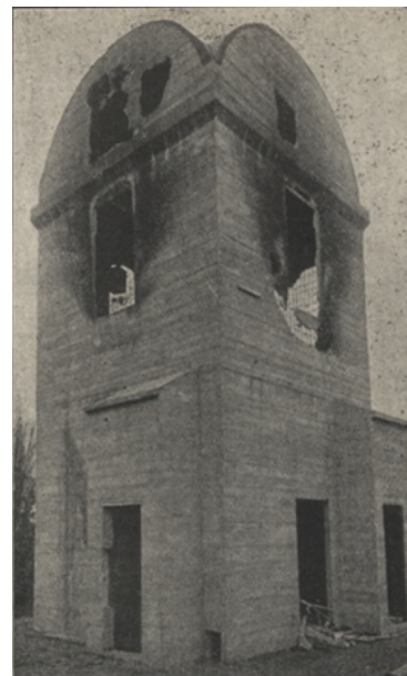
(c) North-east side of the building after the fire on the first floor
