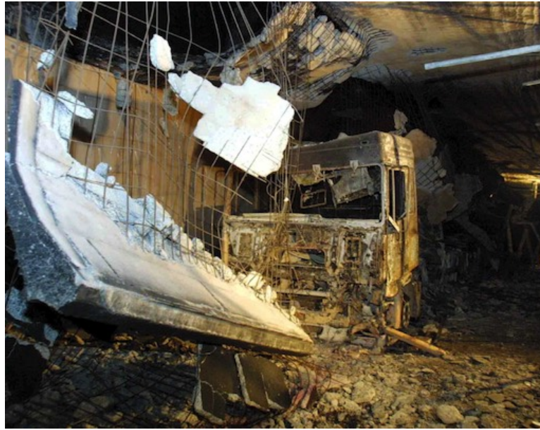
(a) Partially collapsed ceiling (picture by DPA)
