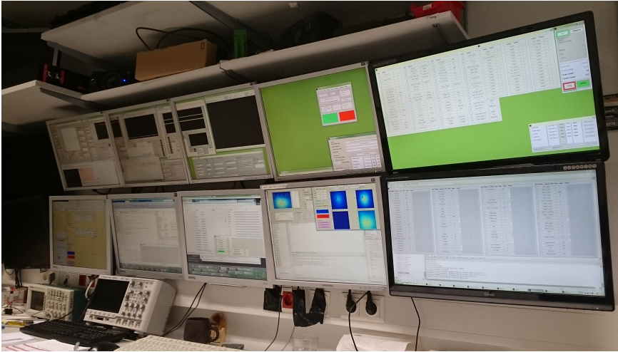
Figure 10.6.: Picture of the control room. Not one screen to many.
