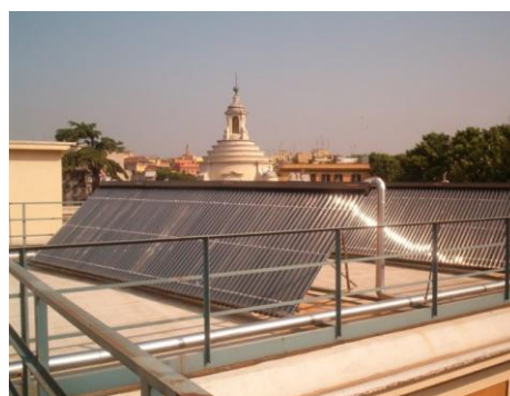
Figure 3.2.4.3: Evacuated Tube Collectors Application (Hotel in Rome, Italy) Source: Renewable Heating & Cooling, European Technology Platform
