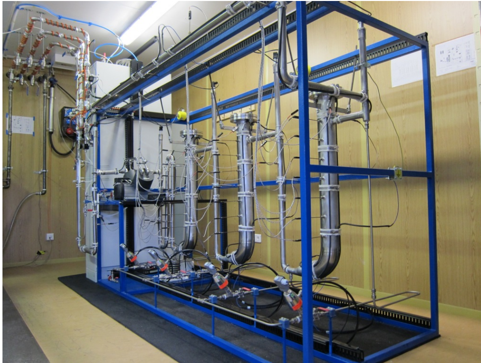
(a) The WGS pilot unit during construction work, prior to heat isolation.
