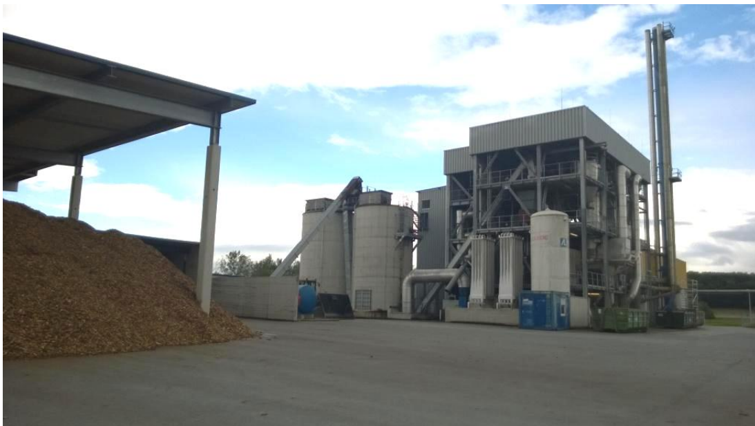
Figure 4.1: Picture of the DFB biomass steam gasification plant Oberwart, Austria in 2014 [7].
