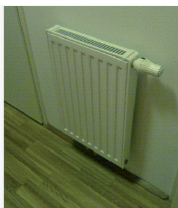
Fig.32 radiator in kitchen/ living area
