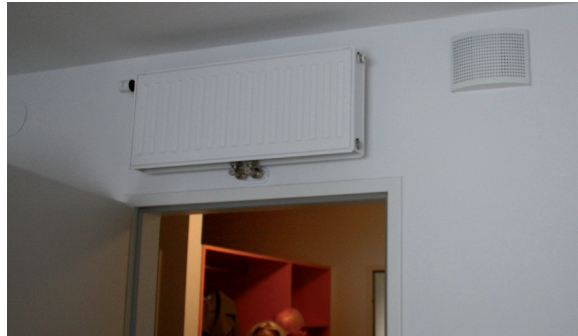
Fig.34 radiator, ventilation outlet and thermostat in bedroom
