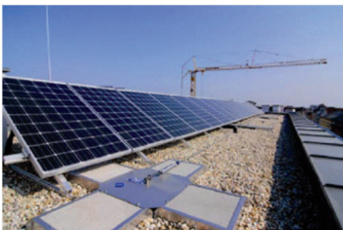
Fig.35 4 kWp flat roof at 30 degrees
