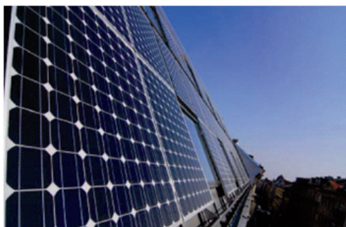
Fig.37 14.7 kWp pitched roof at 58 degrees
