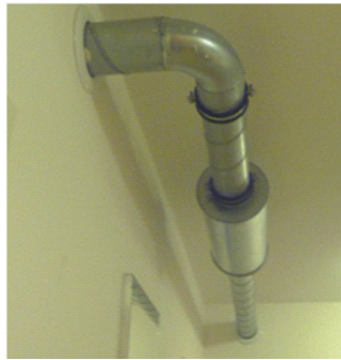
Fig.41 Ventilation System- room partial view.
