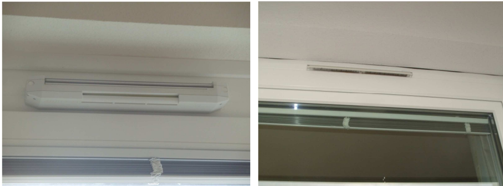
Figure 24: Air inlet of apartment 112
