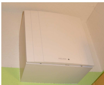
Figure 27: Fan in the bathroom of apartment 112
