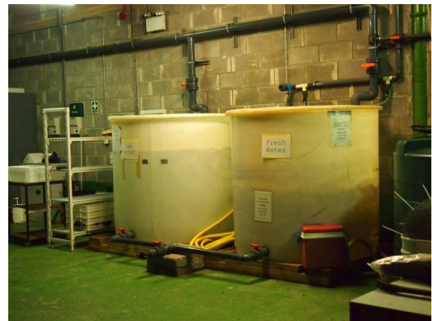
Fig. 5.2.2. Water circulation units.
