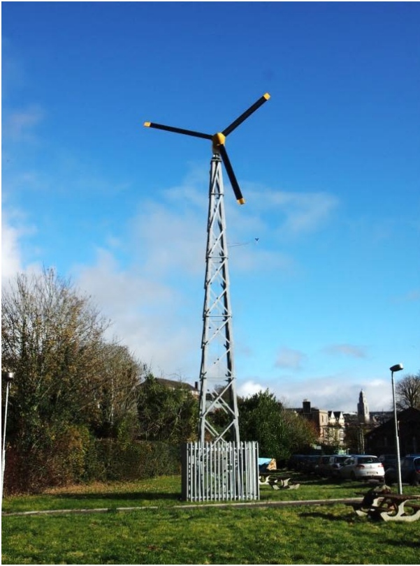
Fig 4.1.2. Bergey Excel 10 turbine on UCC Campus, looking west.
