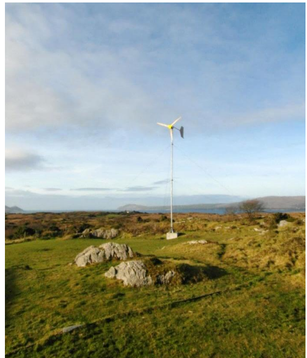
Fig. 4.1.3 Hugh Piggott turbine in Ratooragh near Schull.
