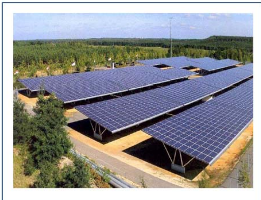
Figure 43: PV Carport at Lausitzring in Germany 61
