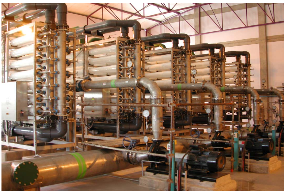
Abbildung 9: New Goreanagab Water Reclamation Plant – Ultra-Filtration
