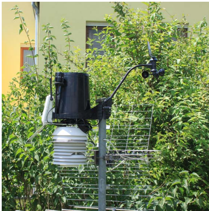
Figure 3-14 Installed weather station at "Kindergarten Pachern"
