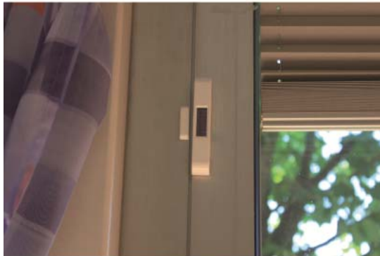
Contact sensor, door to outside, Thermal Zone 7, #CB1
