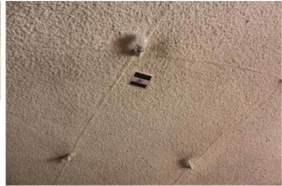
Occupancy sensor, Thermal Zone 6, #MA2
