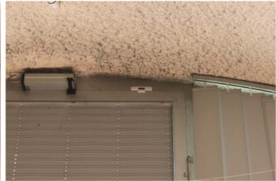
Contact sensor, top window, Thermal Zone 6, #CA3
