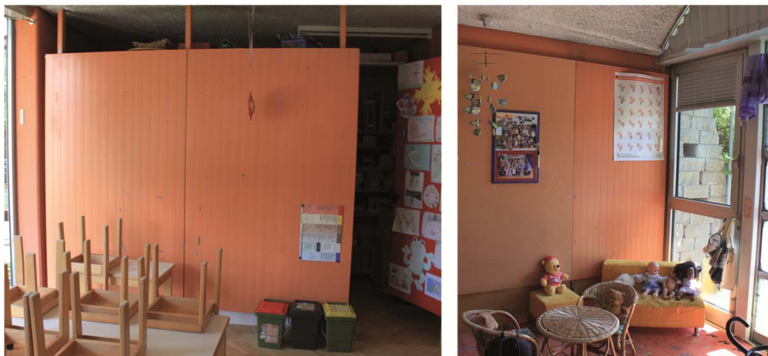
Figure 3-19 Heating panels at "Kindergarten Pachern"
