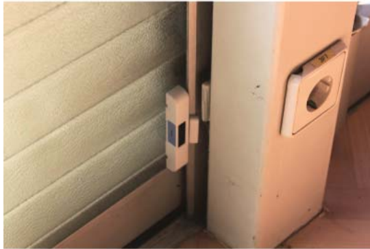
Contact sensor, garage door, Thermal Zone 6, #CA2
